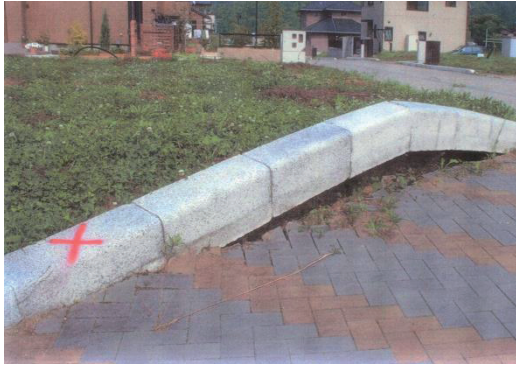
Figure 6 Expansion of concrete block due to DEF [15]
