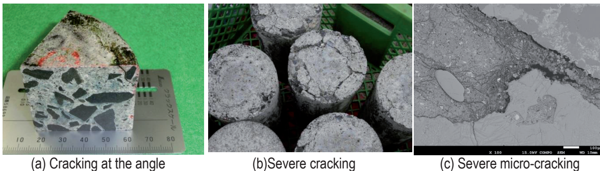
Figure 5 Cracking of concrete subjected to wetting-drying cycles of seawater with large temperature variations
